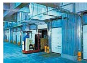
Cold storage warehouse
